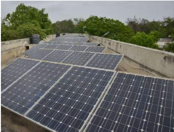
80 kW Solar Power Plant in Raj Bhawan
