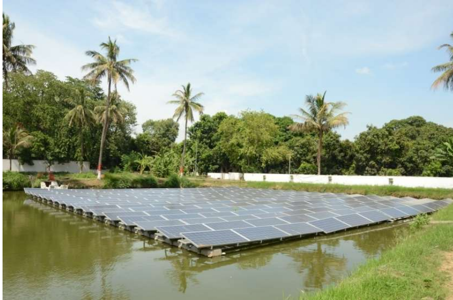
Solar Panel in the Pond for Street Lighting
